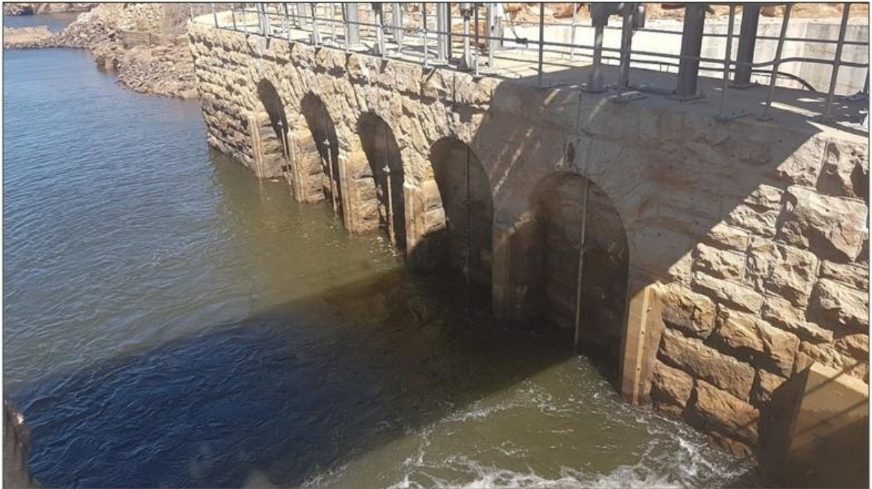
Figure 13-4: Bulshoek Weir outlet structure sluice gates
